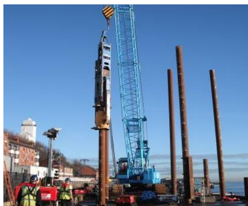
Figure 8: Photograph illustrating an Impact Hammer driving and setting the Steel Tubular Pile to its design parameter.
